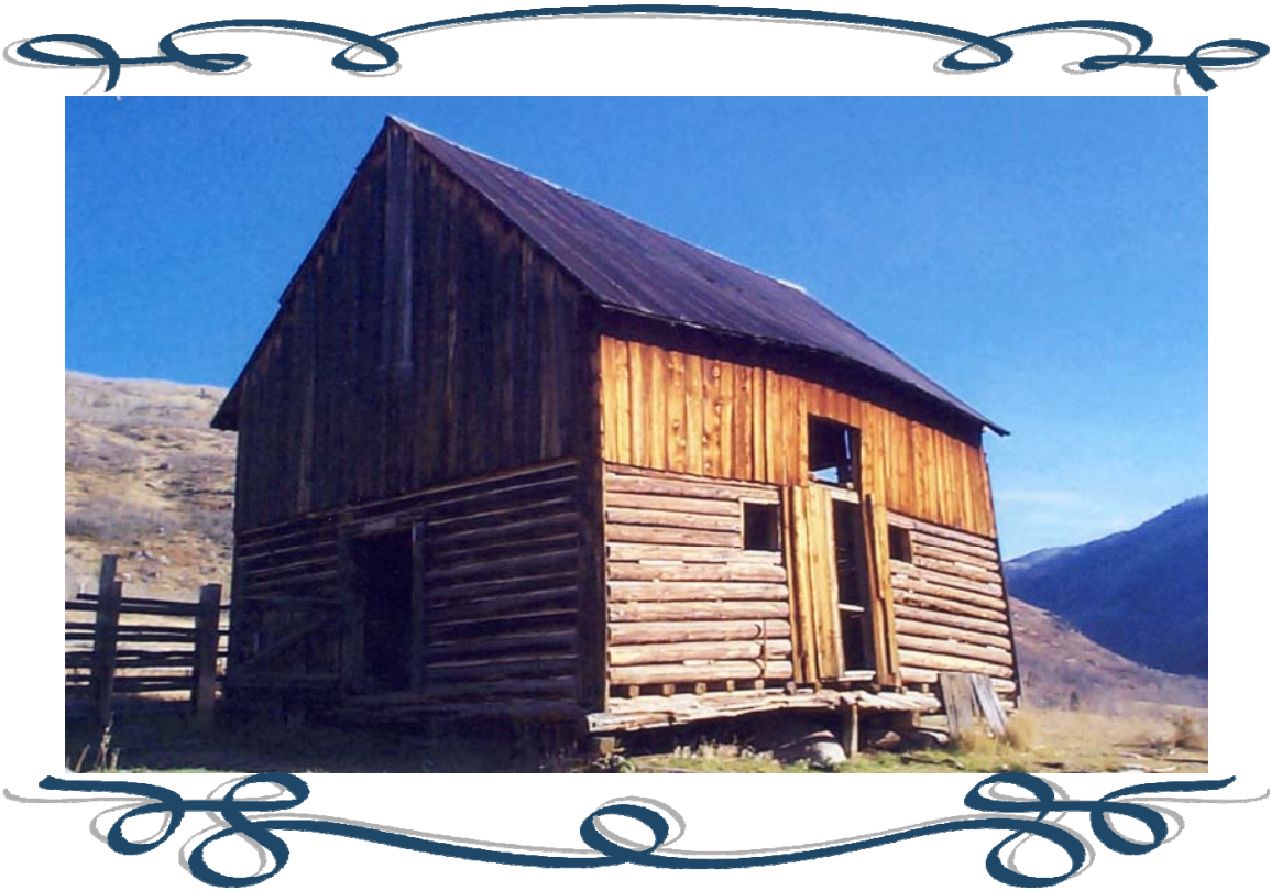
A, & C. MAD CREEK BARN, Mad Creek Ranger Station Routt National Forest; trailhead off County Road 129, North of Steamboat Springs
